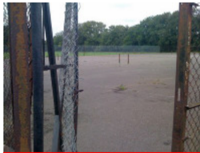
Rusting broken tennis court gate
